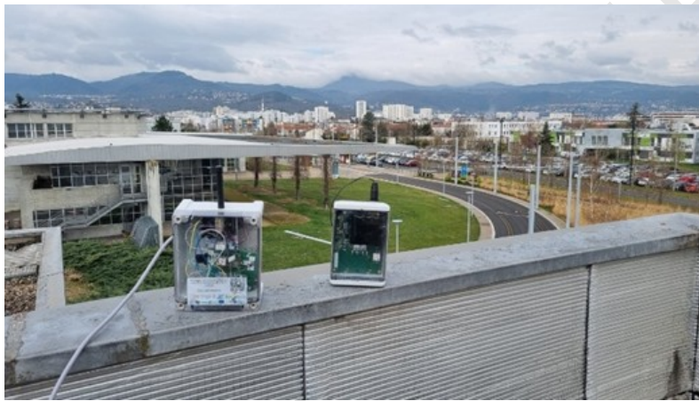
Figure 8: Satellite modules installed in the roof of the laboratory located on the campus of the University Clermont-Auvergne
